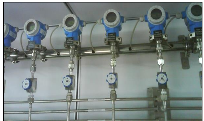
Fig 1: Pressure transmitter installed in an industrial process plant
