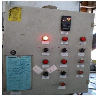
Fig 3: Control panel and boiler activation.
