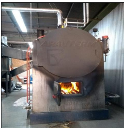
Fig 2: Boiler in operation.
