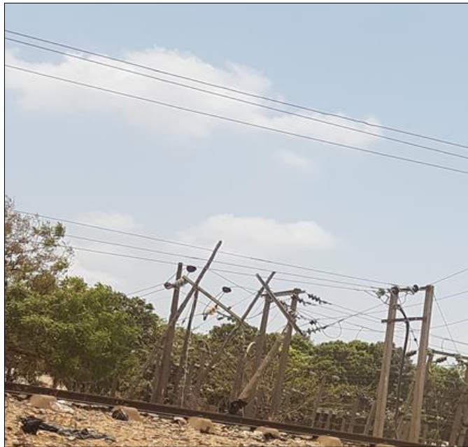
Fig 2: A Transmission Line Exposed to Risk (North-West) Nigeria
