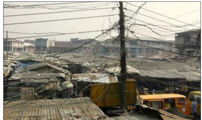
Fig 1: A Distribution Line Exposed to Risk (South-West) Nigeria
